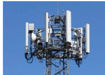
5/6G Base station
